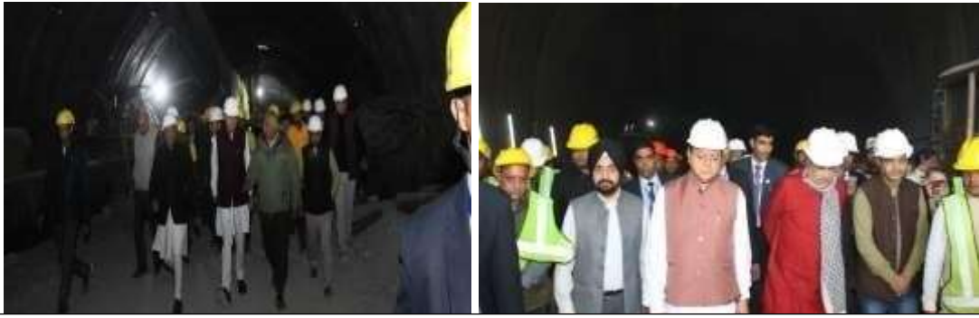
Site visit and monitoring of progress on evacuation process of trapped workers
