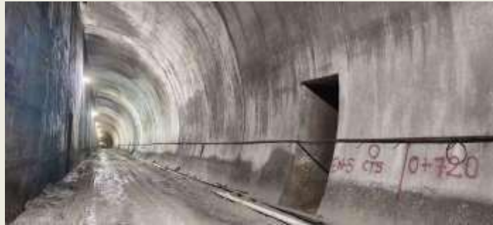
Silkyara Tunnel before the incident
