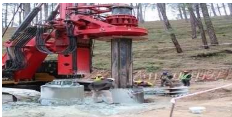
Vertical Drilling on the roof of tunnel for alternative rescue of workers
