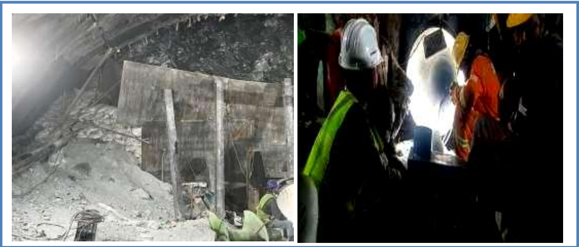
Fortification of the mouth of collapsed section for safety and gas cutter to remove auger machine
