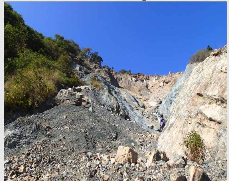
Loose debris covers the bed rock
