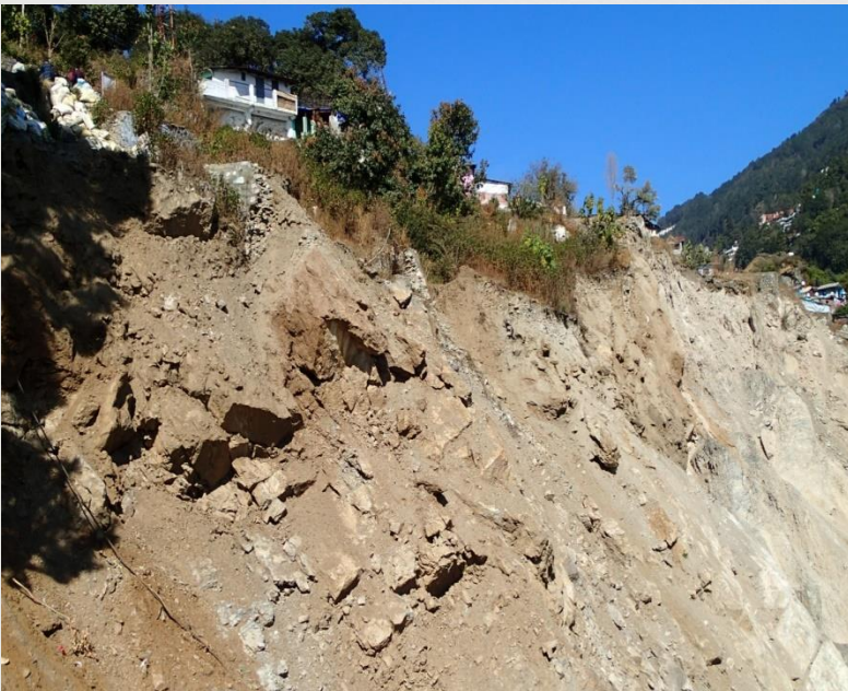
Scarp of failed slope - Loosely held
