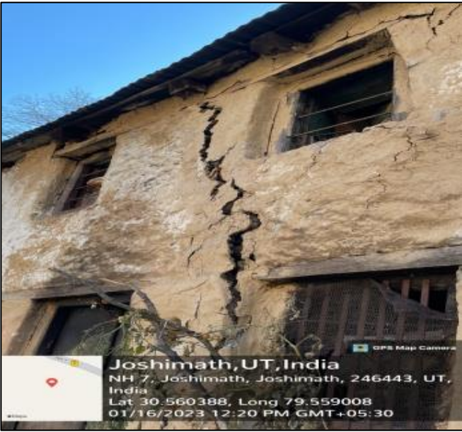
Vertical shear crack along the wall
