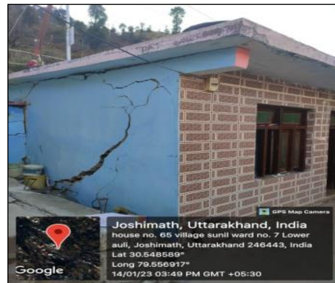
Failure of masonry infill
