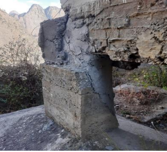
Shear Failure at column footing junction
