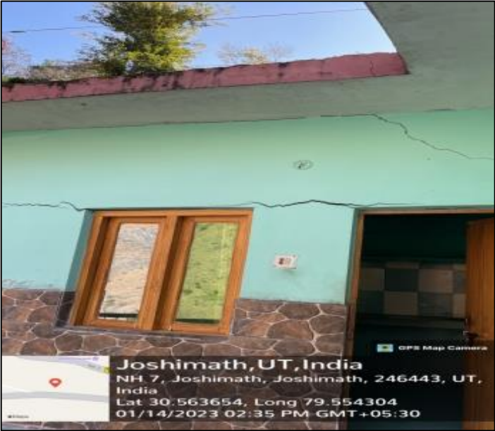
Sliding Shear Failure of Masonry Building
