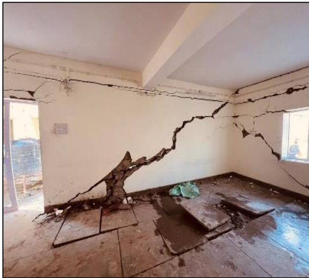
Failure in Masonry building
