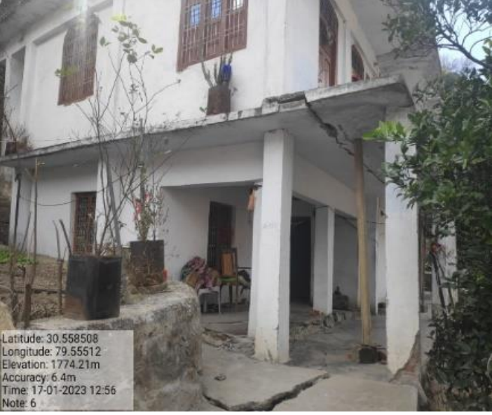
Excessive cantilever projection
