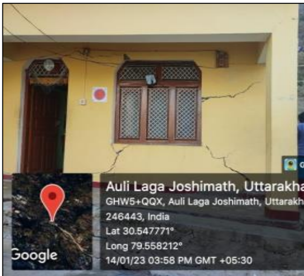
Diagonal shear Failure of Masonry Infill
