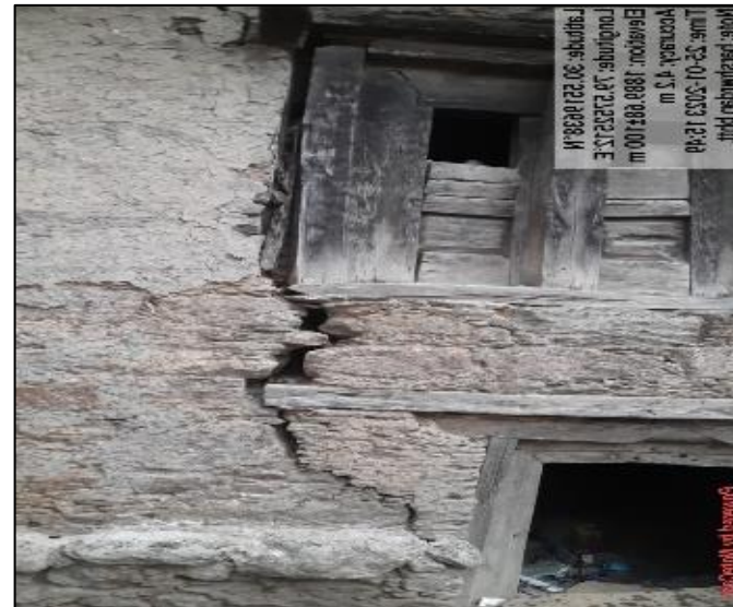
Failure of rubble masonry
